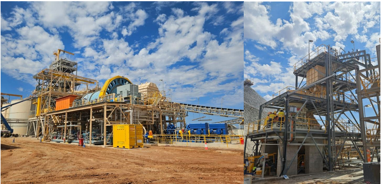
Figure 5: Ball mill installation (LHS) and new pebble crusher (RHS)
