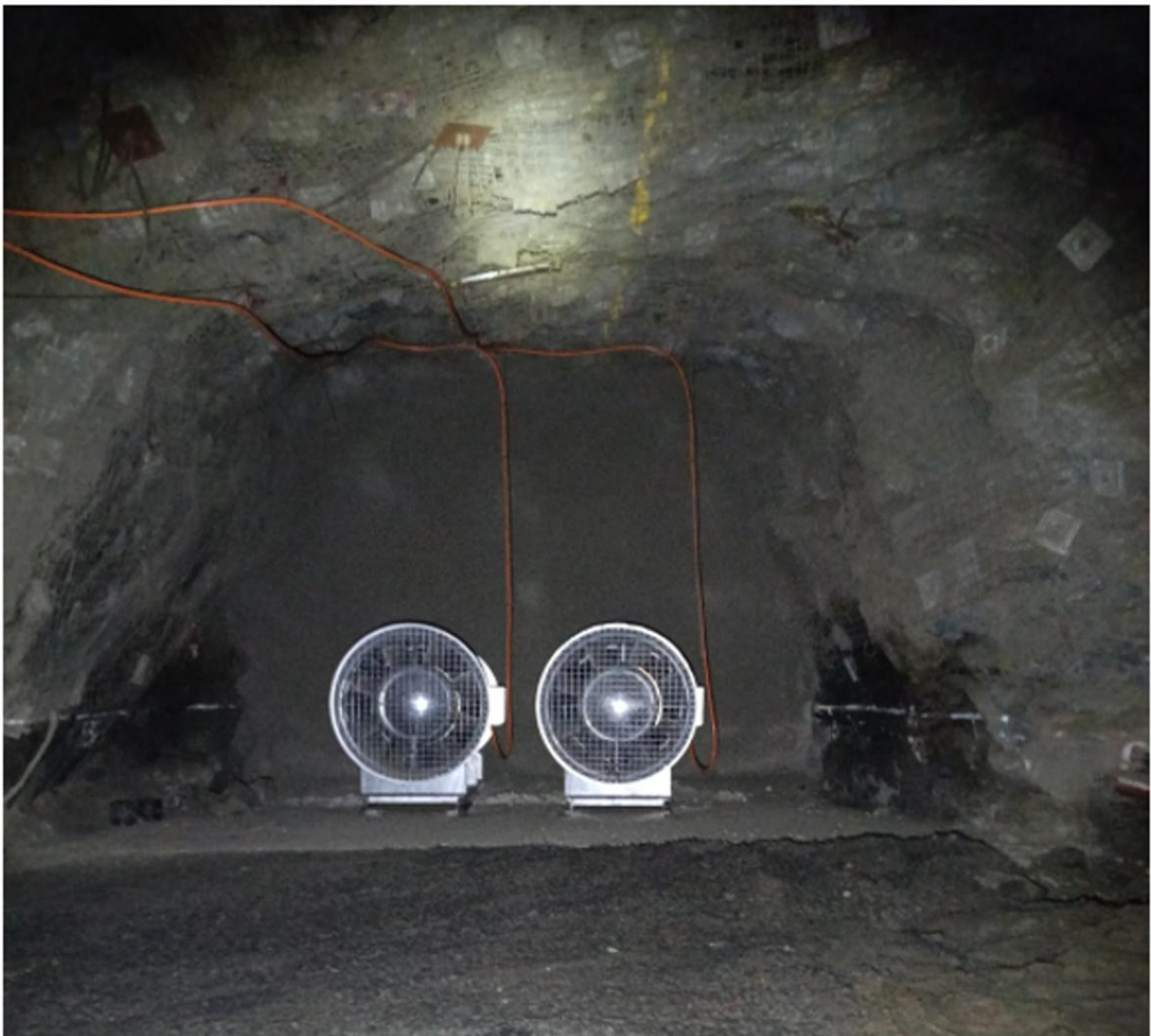
Figure 5: Primary ventilation fan installation at the Pinnacles underground workings.
