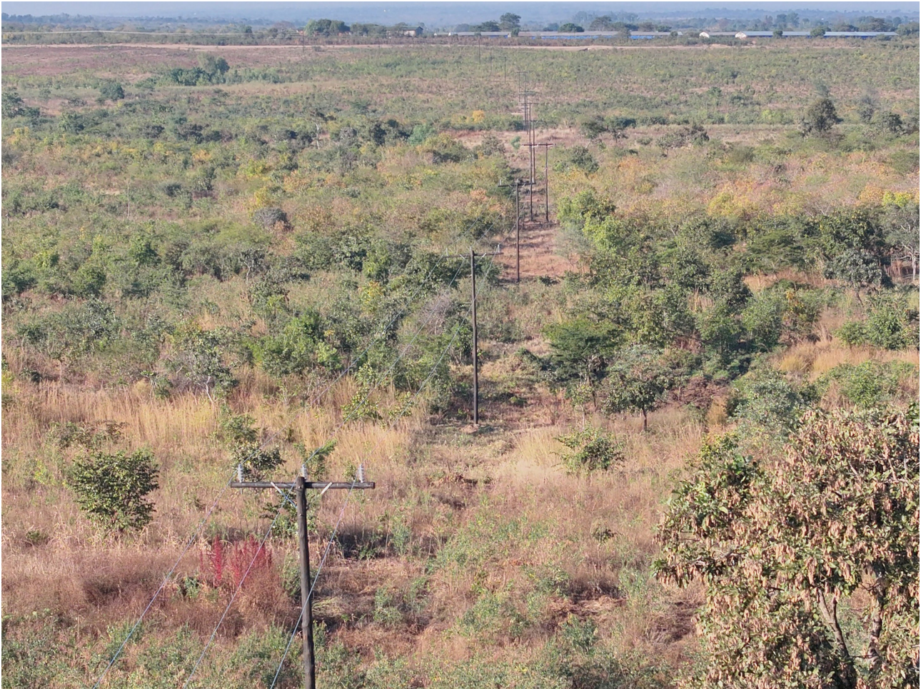
Picture 2. Kangankunde's dedicated 33 kV transmission line, forming part of the 27 km grid connection from Chingeni Substation to the Project site. The line has now been commissioned and successfully energised.
