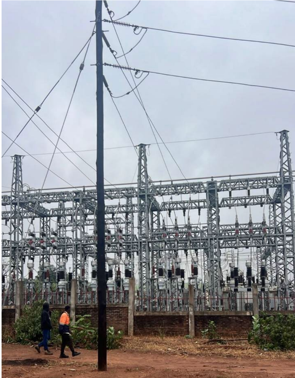
Picture 1. Chingeni Substation, the connection point for Kangankunde's dedicated 33 kV grid supply. The 27 km line to site has been inspected, commissioned and successfully energised by ESCOM.
